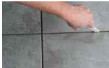
9. Install ARDEX Grout in accordance with the relevant datasheet. Ensure grout booster is used.
