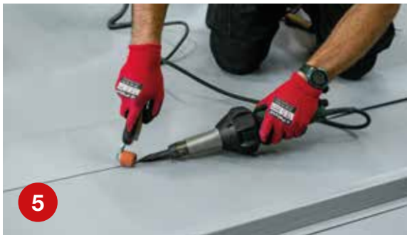
5 Hot-weld the membrane cover strap which should be 180mm in width to seal over the fixing line, taking pressure off the existing membrane.
